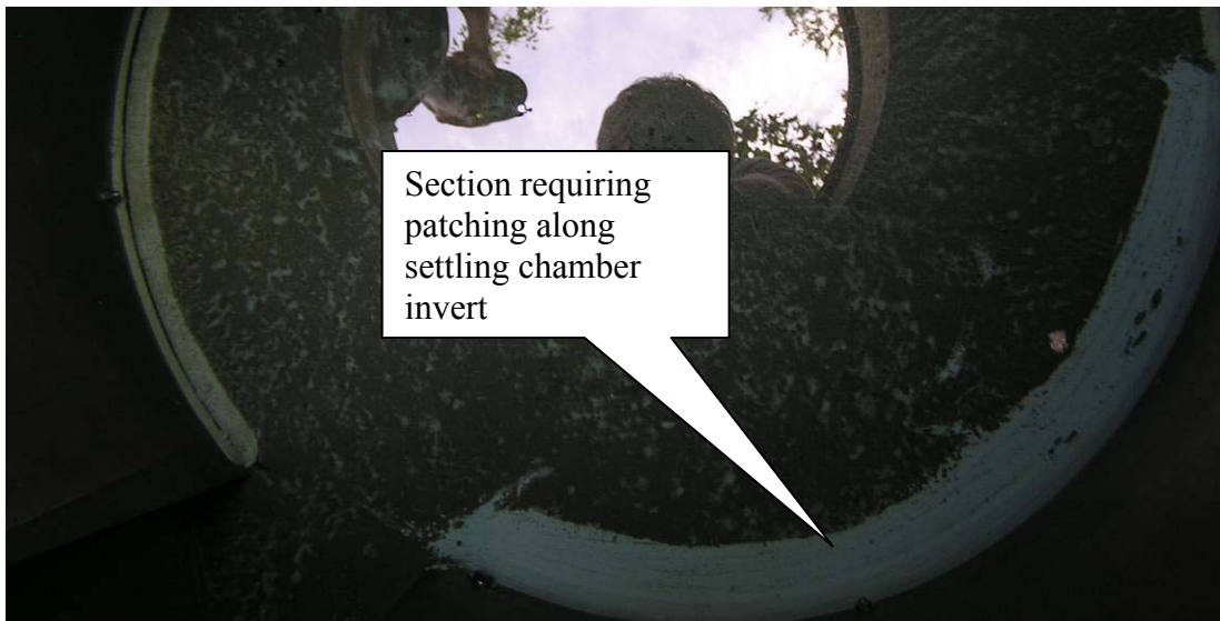
Figure C.16: View of the base of the stainless steel cylinder serving as a swirl chamber and new sealant applied (thicker section along lower right) to minimize improper hydraulics.
