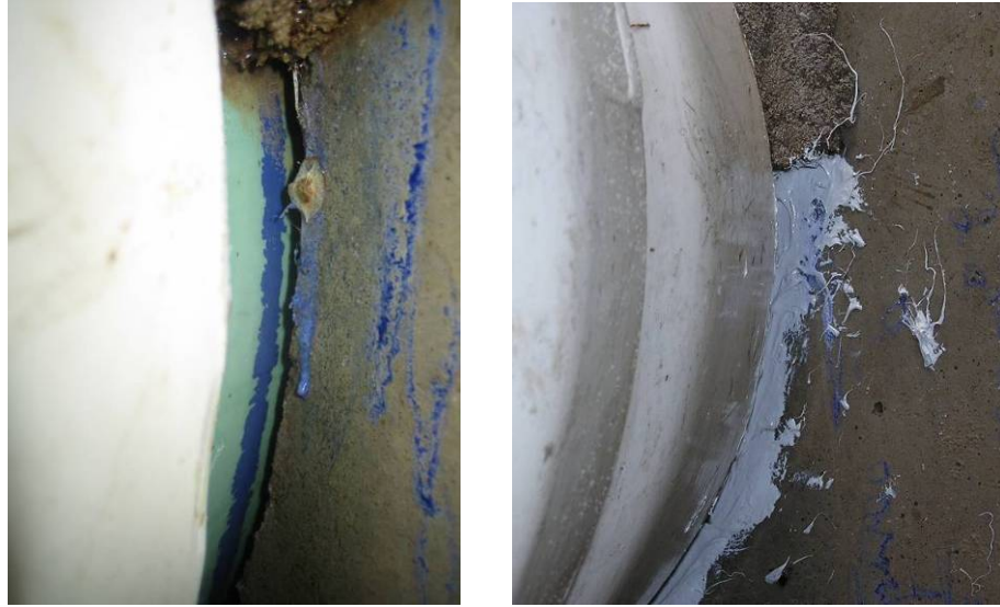
Figure C.8: (Left) Water was initially able to flow between treatment manholes through an approximate 1.3 cm ( ½ in) gap between the PVC pipe and concrete manhole wall. (Right) The leaking gap was patched with Vulcum polyurethane to ensure proper system hydraulics.
