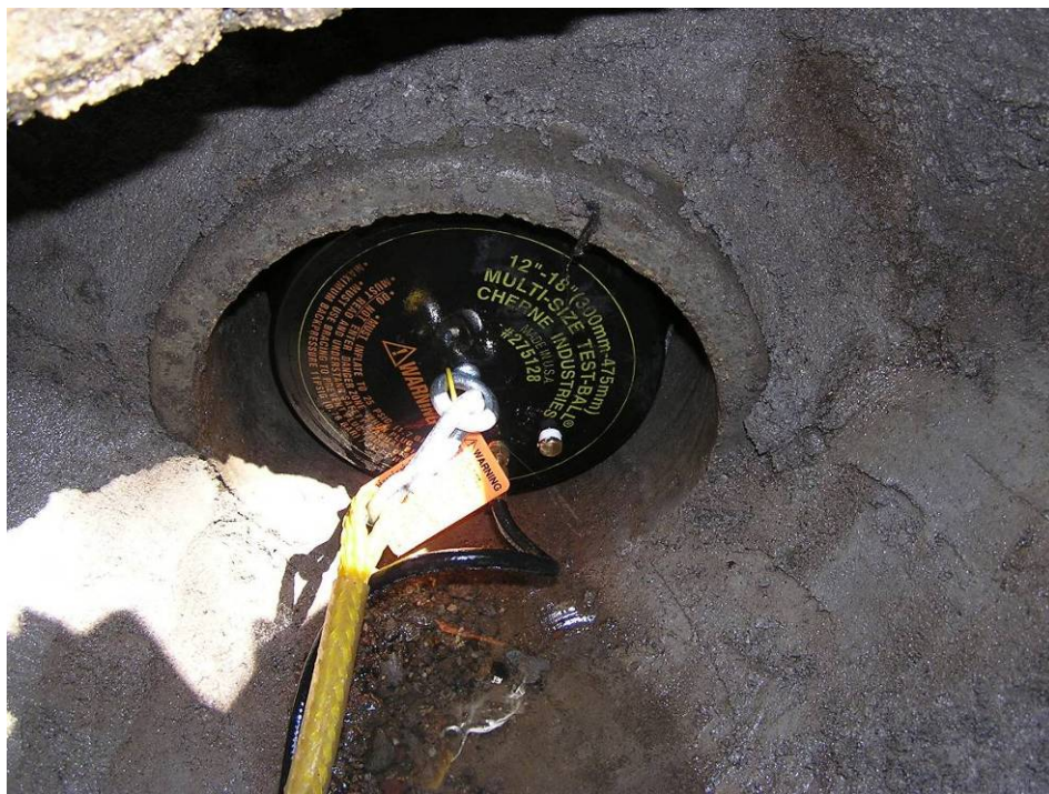
Figure C.13: 12” diameter inflatable plug loaned by the City of St. Louis Park Public Works for use at CBMH4 as shown in Figure C.12.
