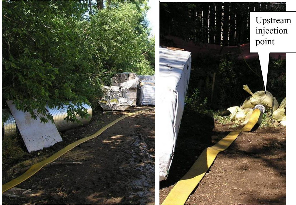
Figure C.12: Depiction of 4 inch fire hose used to span about 150 feet from the hydrant (not shown, see Figure C.11) to the influent injection point (right).
