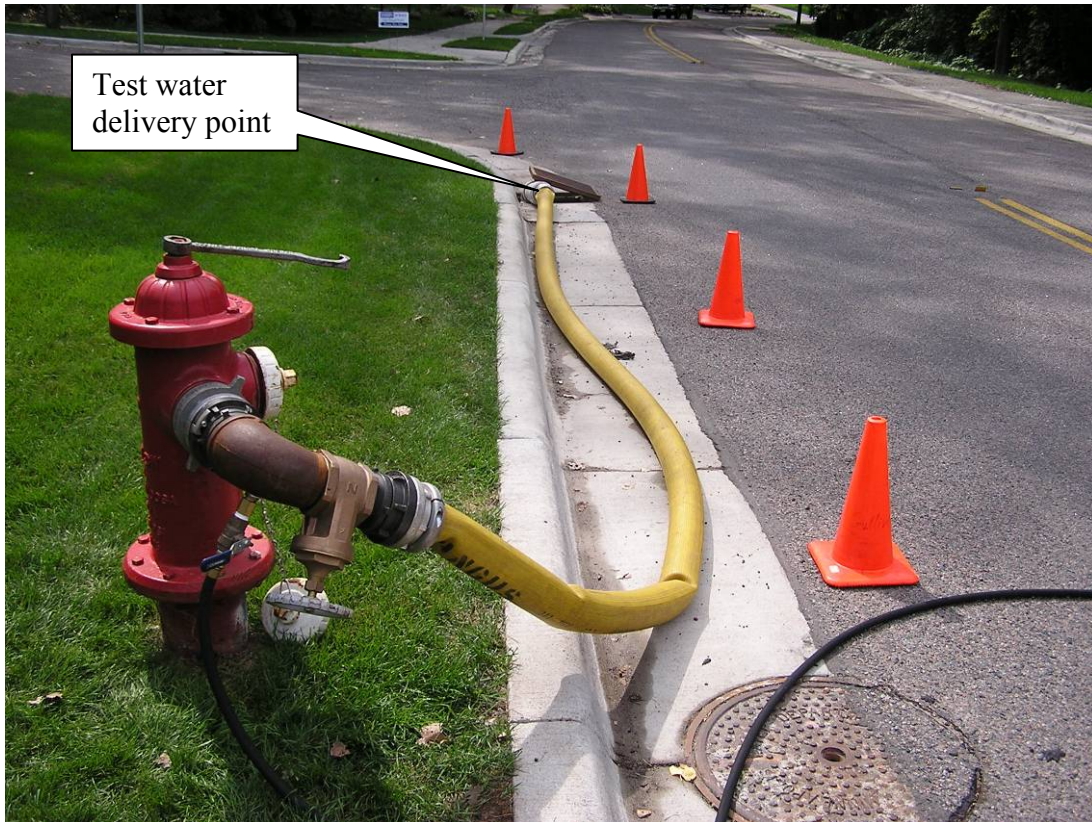
Figure C.24: Influent piping system from hydrant to catch basin for CDS testing.
