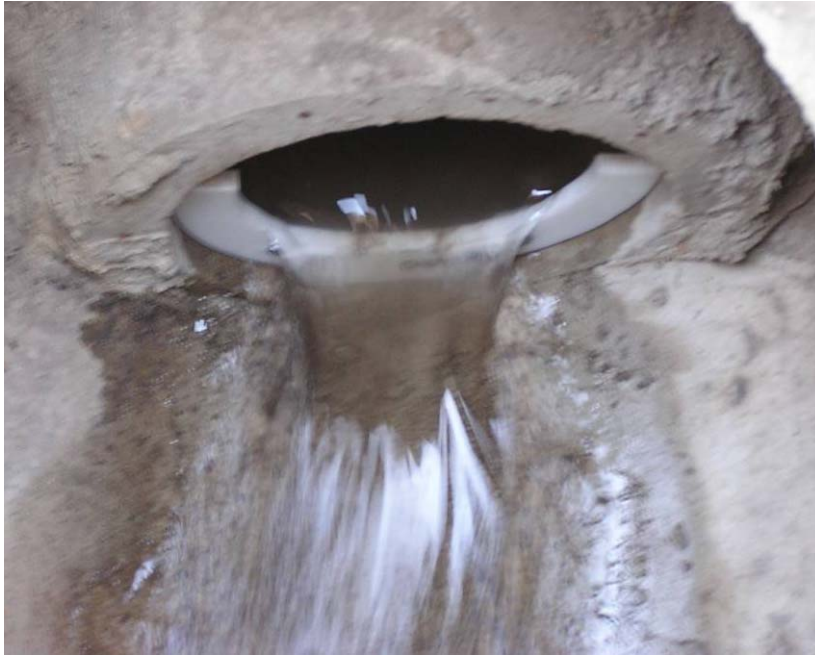
Figure C.10: Pre-calibrated 12” circular weir installed downstream of the Vortechs System. Pressure transducer and transducer anchoring not shown. This weir location provided free outfall conditions at all flow rates due to the favorable gradient across the manhole and downstream storm drain system.
