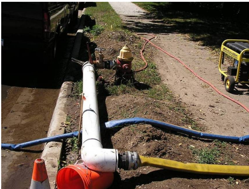
Figure C.11: Upstream portion of influent delivery system from the water source at the hydrant to the first reach of 4” fire hose in the foreground.
