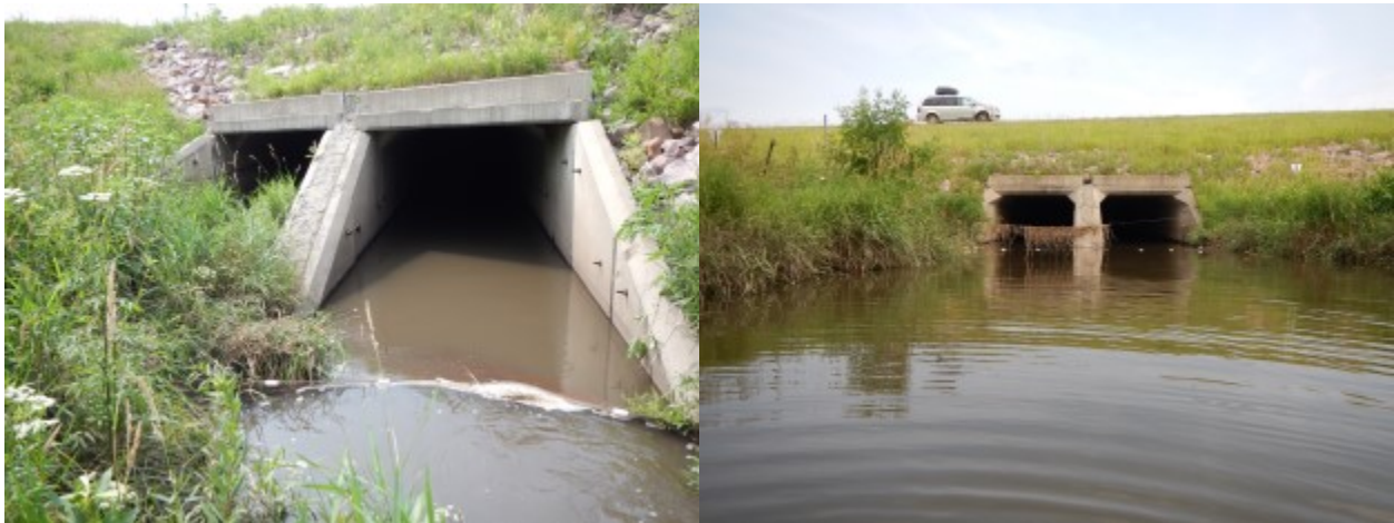
Figure 2.6 Upstream view of culvert 8884 on Split Rock Tributary, Rock County, showing vegetation in left barrel (left) and downstream view of culvert 8884 showing large pool with surrounding vegetation.
