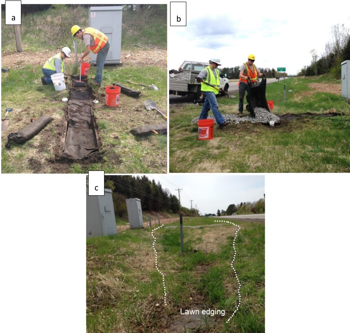
Figure 4.1. Maintenance performed at the ditch check site in May 2017. The topsoil and sod covering the filter insert section were removed (a & b), and lawn edging (highlighted by white dashed line) was installed along the ditch check (c).
