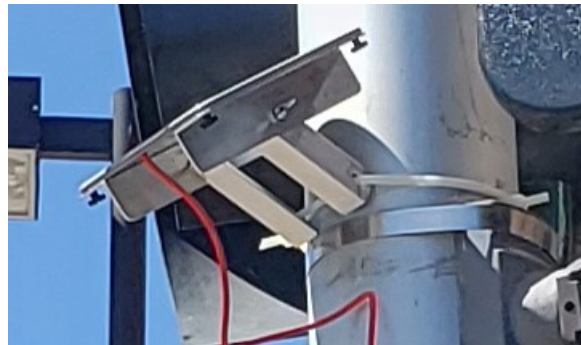
Figure 2.9 A Solar Panel with Mounting Assembly on a Signal Pole.
